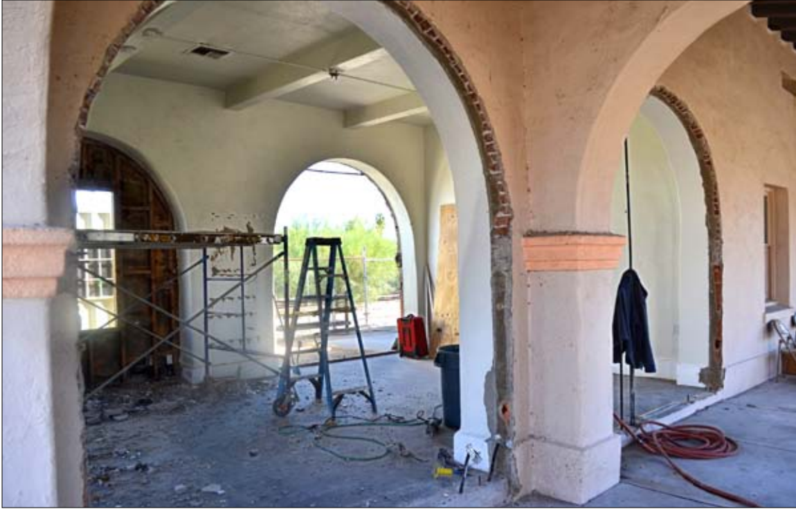
Demolition and remodeling work on the historic Depot in the Plaza is well under way, with the north side arches being opened up to restore the original open-air waiting area. Crews are working at the other end of the building to even up the floor levels. Project supervisor Kirk Havermahl of G&G Construction said work is going smoothly.
