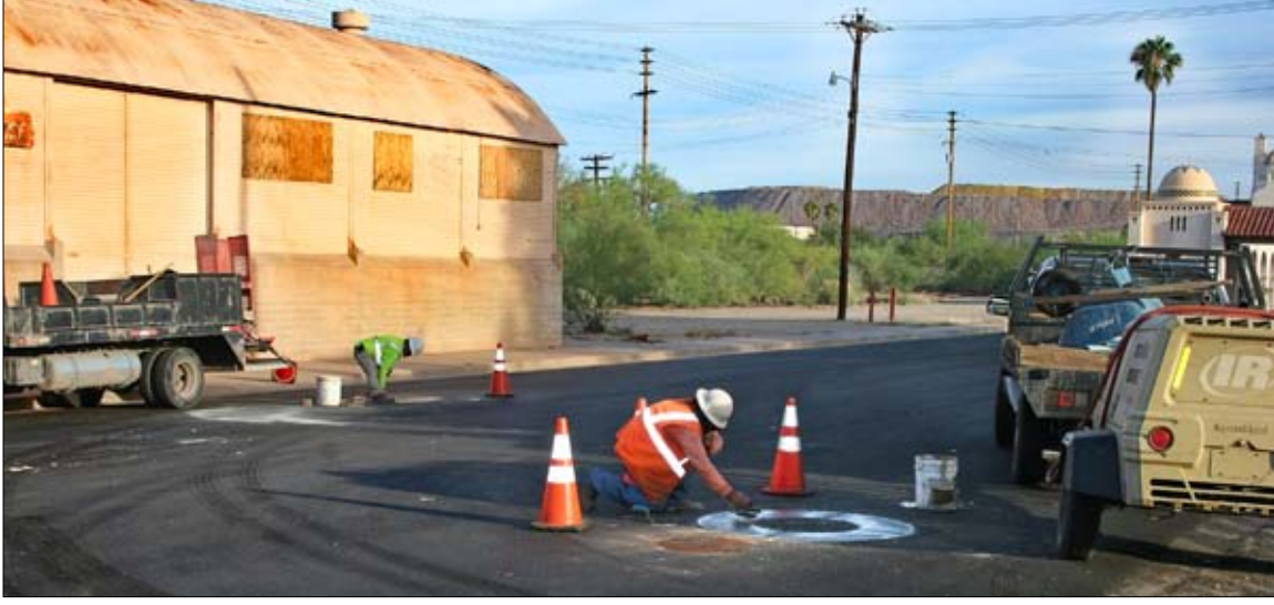
Workers put the finishing touches on freshly poured concrete around manhole covers in the new asphalt behind the Plaza. Smooth, black streets are gradually taking the place of the potholed and cracked roadways that were patched after utility line upgrades crossed their paths.
