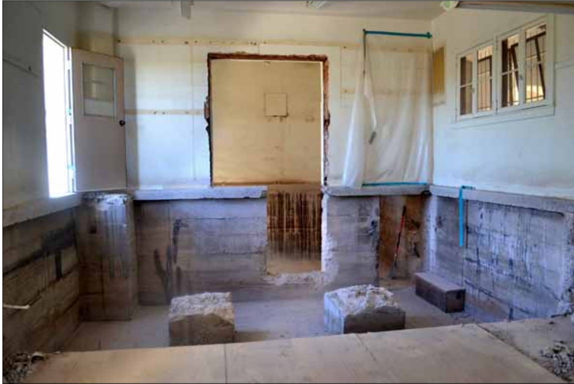
The demolition and rehab work continues at a fast pace at the historic Ajo Depot, as seen in this picture of the north end interior. What was formerly a partial basement area used for baggage and other storage is being leveled to make it totally accessible in its new use as a visitor's center.
