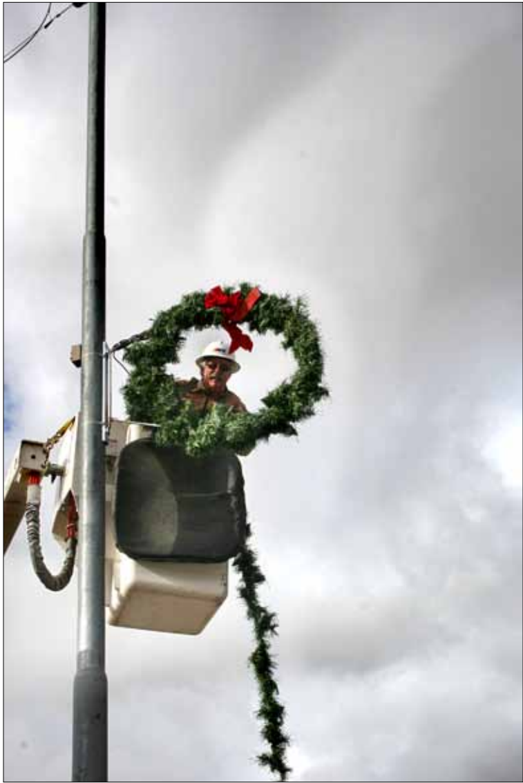
Local lineman Scott Boyd of Arizona Public Service picked a cold and blustery Thursday afternoon to install Christmas wreaths on streetlight poles along North Second Avenue. Crews from Ajo Improvement put up wreaths in their service area.
